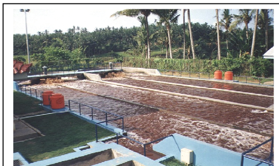
Waste Water Treatment Plant PT. Sinar Sosro - Bali
