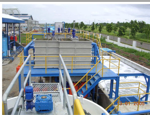
Waste Water Recycle Plant PT. Chemco Harapan Nusantara –
